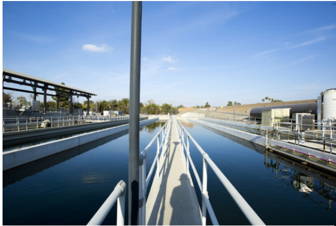
Chlorine contact basin at IRWD MWRP.
