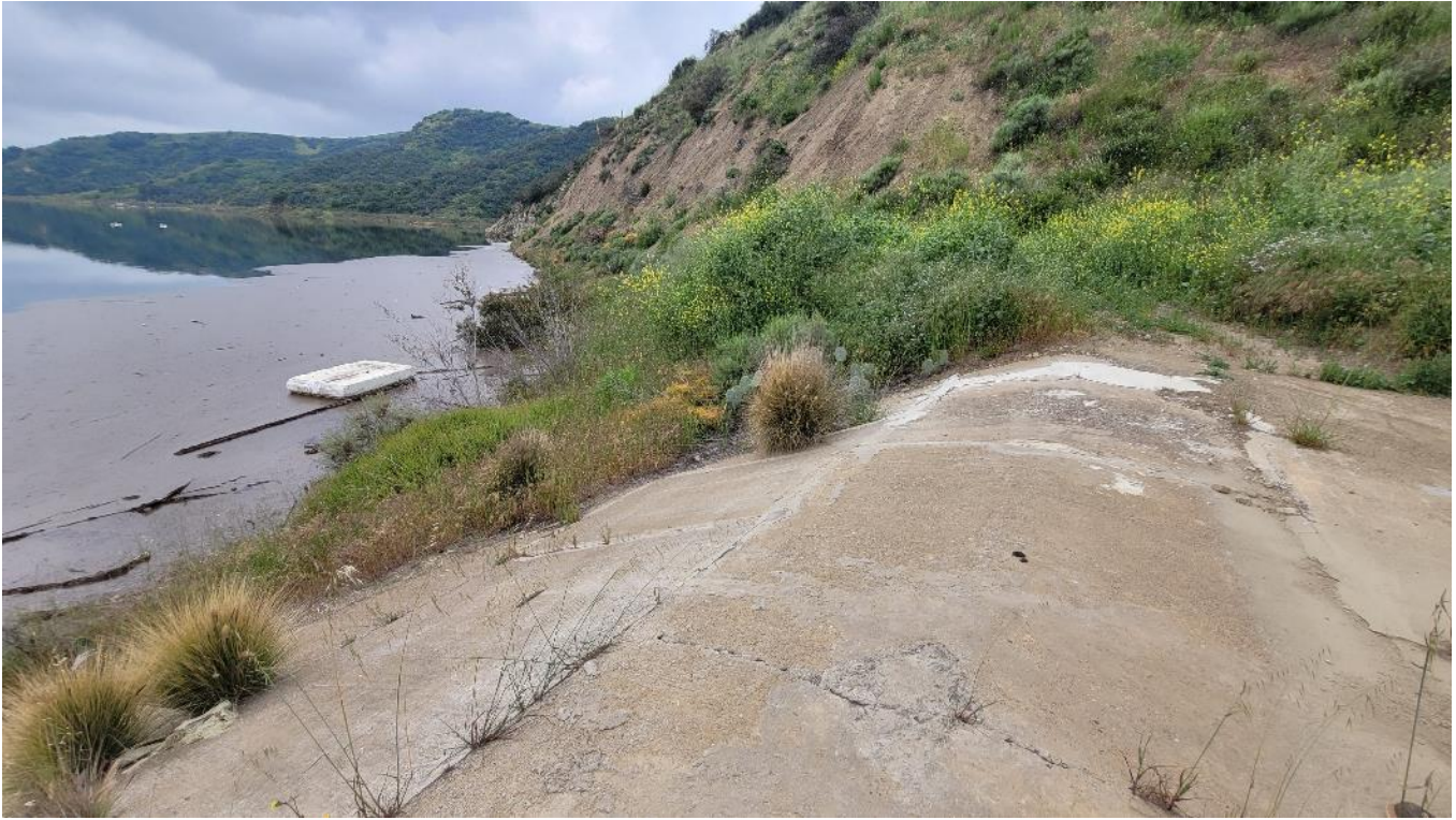
Photo 6: View of the spillway approach with sediment and vegetation buildup.
