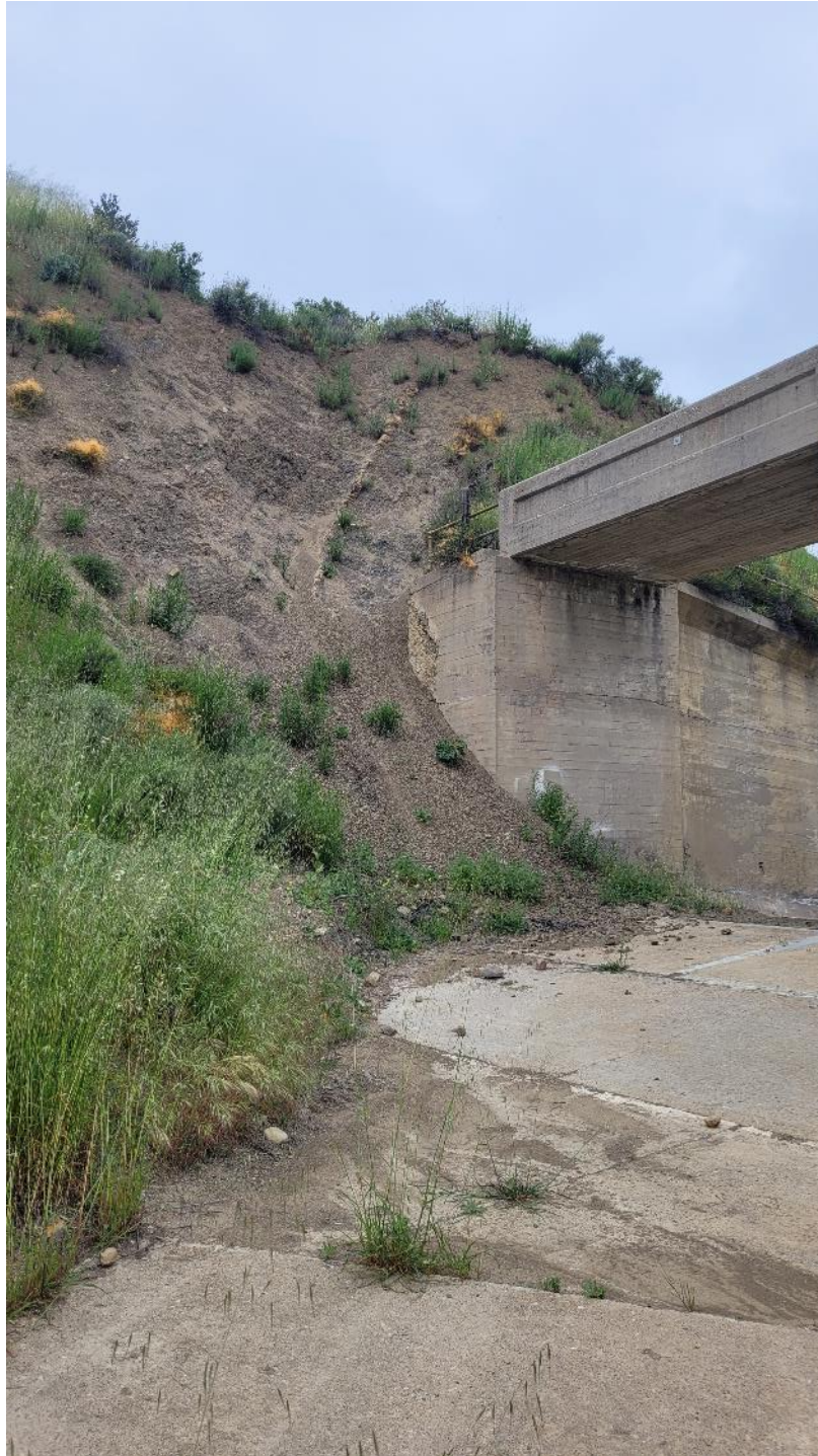
Photo 3: View of the erosion left of the spillway.
