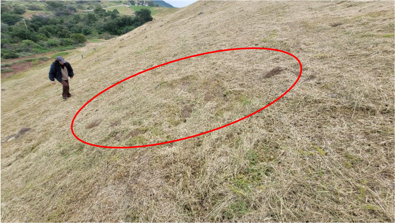
Photo 1: View of new rodent activity along the downstream slope.
