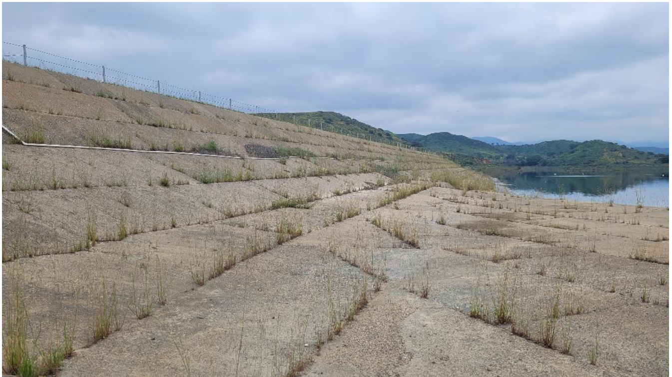
Photo 2: View of the upstream slope with weed growth.
