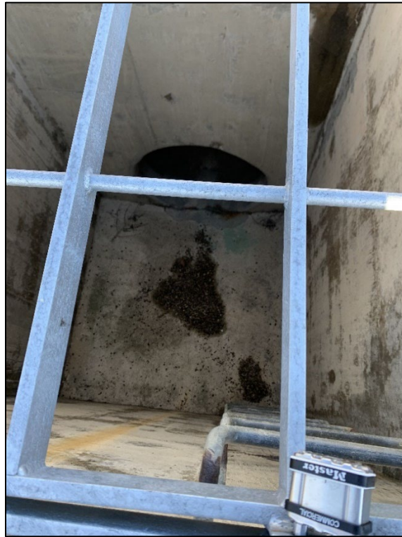
Photo 19) Bottom of left spillway drop inlet structure leads to a 48-inch spillway pipe that discharge at the dissipator structure located at the downstream toe of the dam.
