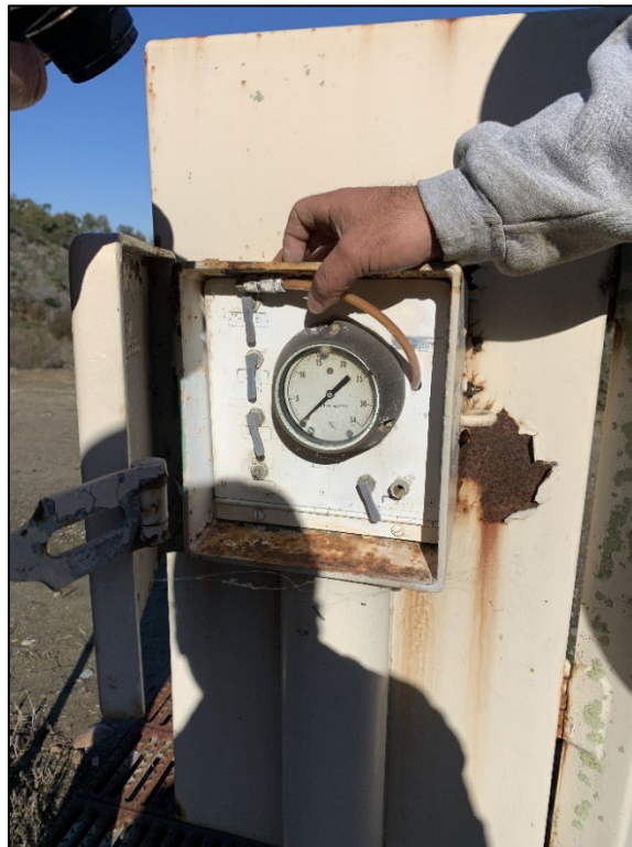
Photo 12) Relief valve gauge behind pneumatic piezometers. Note significant corrosion throughout vault box.
