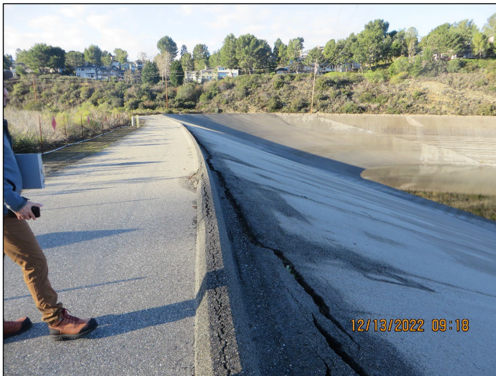
Photo 16) Looking at the southwest corner of the reservoir. Note reservoir line separation cracking and traverse cracking.
