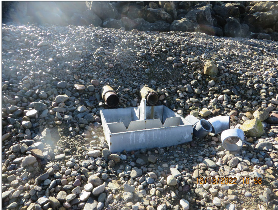
Photo 21) V-notch weirs measuring seepage flows from the Upstream Collector Drains #1 and #2. Note significant corrosion on the drains.
