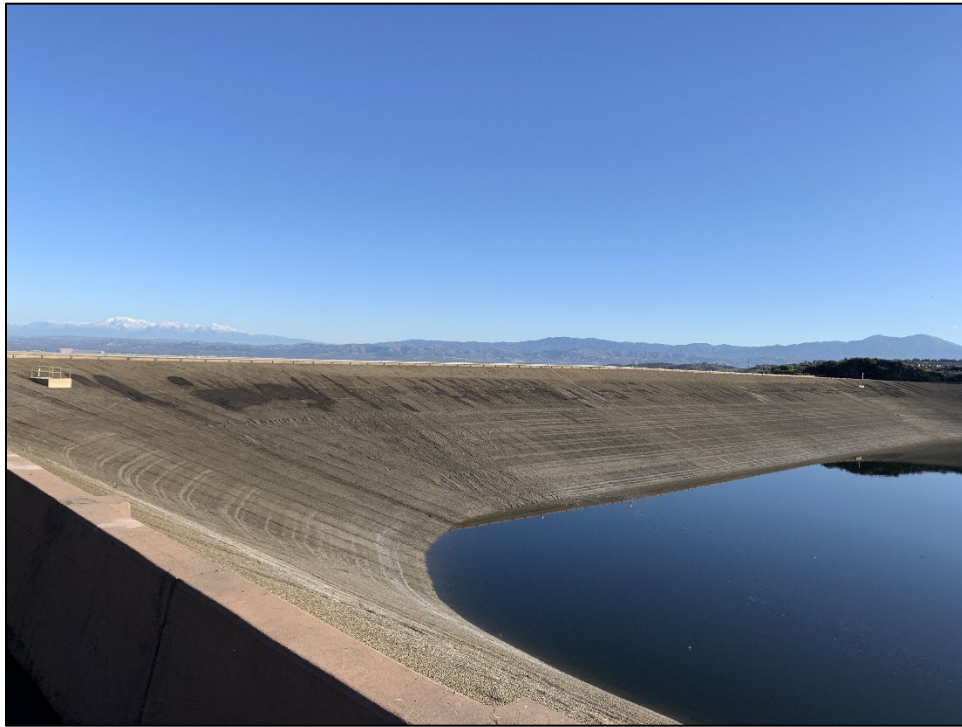
Photo 1) AC-lined upstream face looking towards right abutment. Note the recent patch work.
