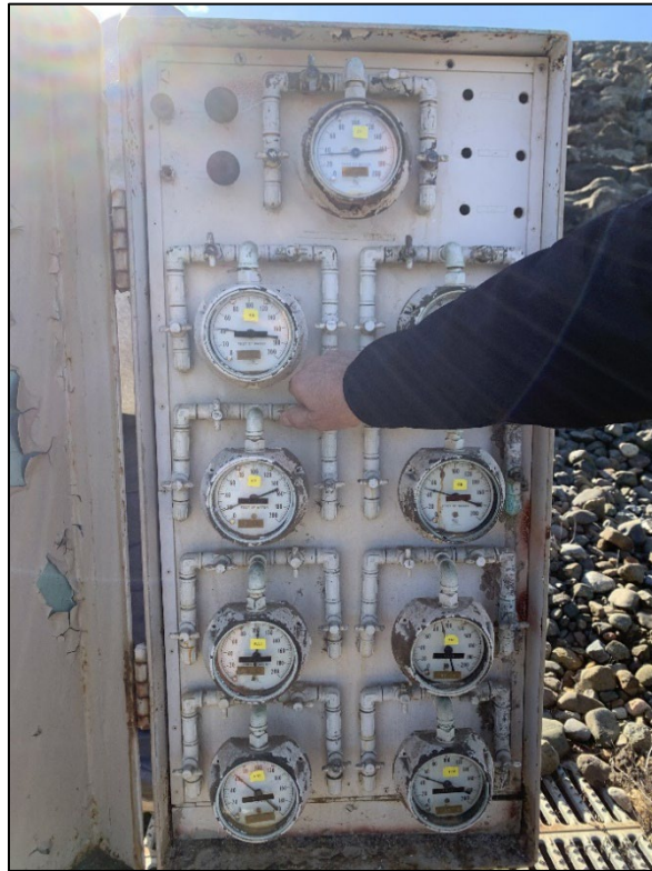
Photo 11) Exercising pneumatic piezometer control valve. Note significant corrosion throughout vault box.
