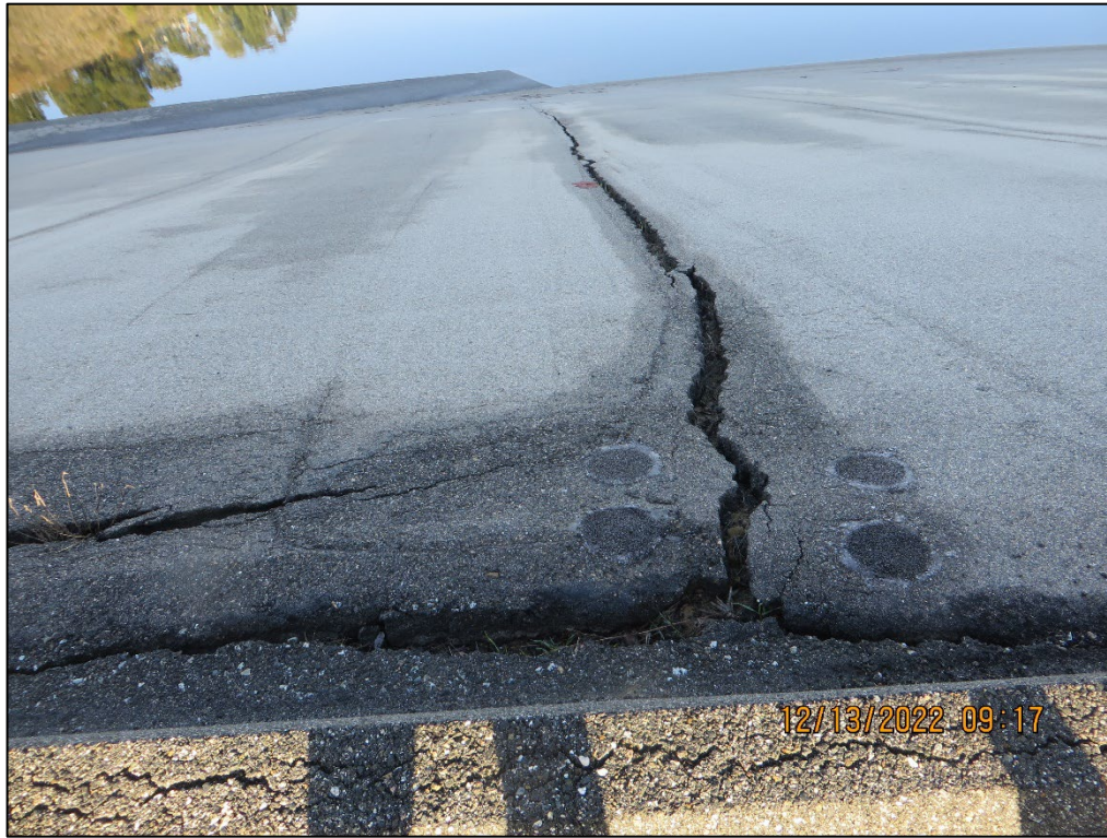
Photo 17) Longitudinal cracking of reservoir liner at the left south end of the reservoir.
