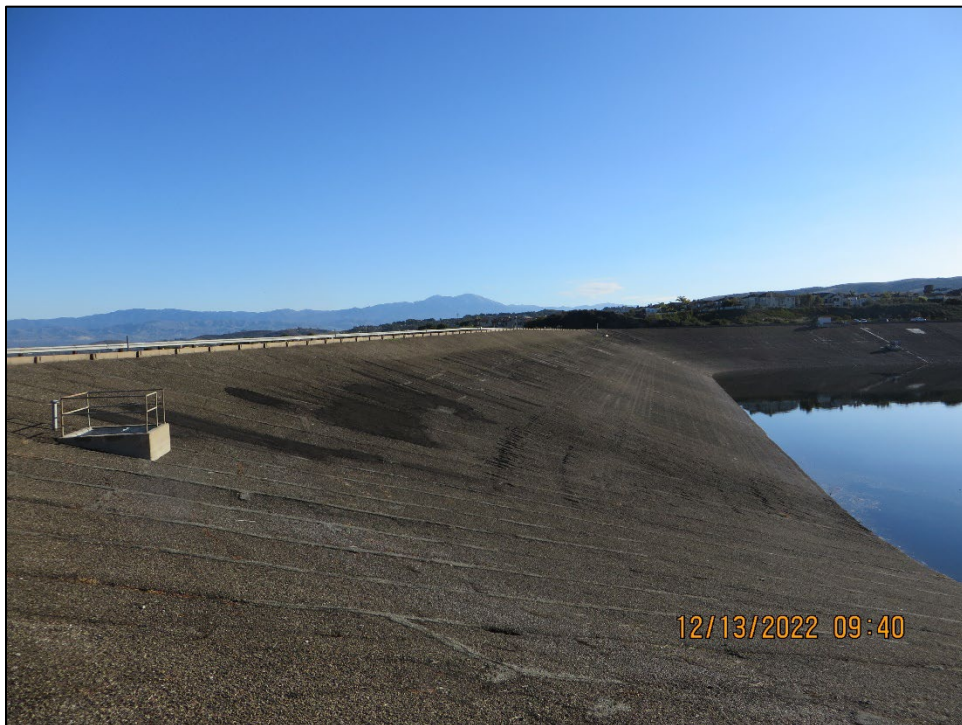
Photo 2) AC-lined upstream face looking towards right abutment. Note the recent patch work.
