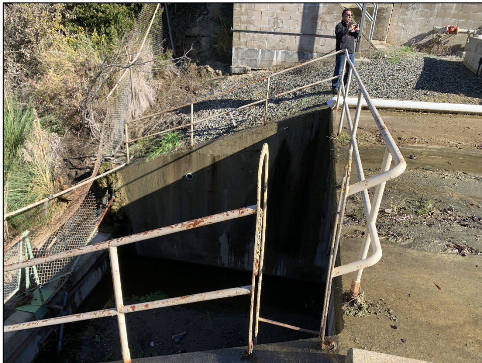
Photo 14) Energy dissipator structure. Note significant corrosion on handrails and ladder.
