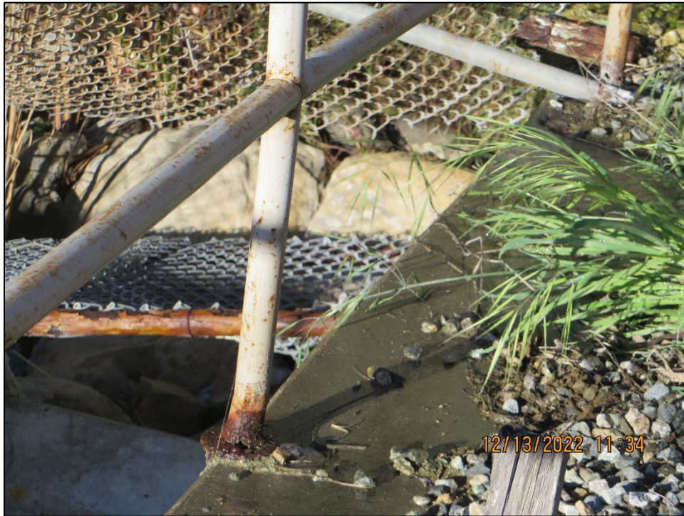
Photo 15) Significant corrosion of safety handrails at energy dissipator structure.
