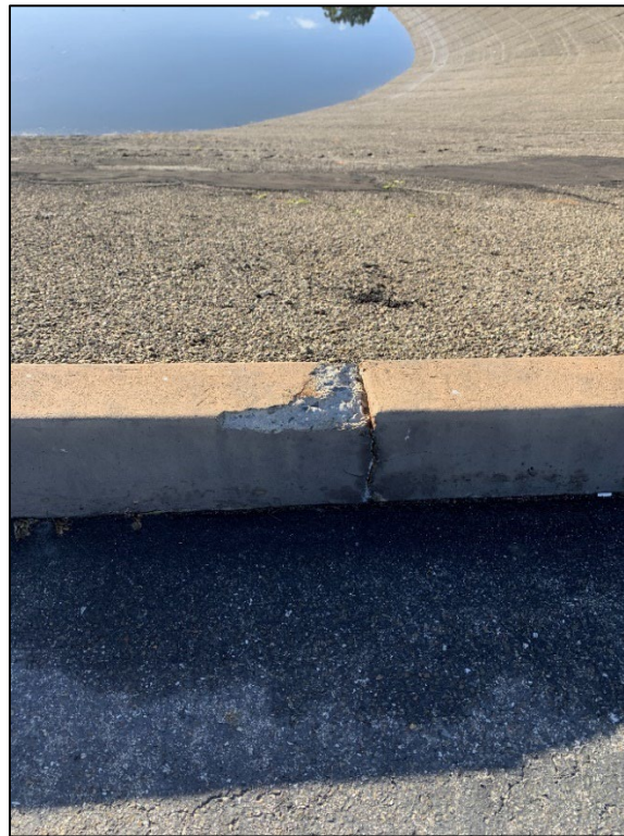
Photo 6) Cracking and spalling at joints of concrete crest curb on upstream side.
