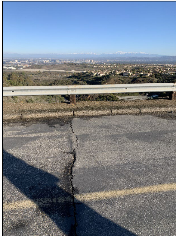
Photo 5) AC pavement cracking looking downstream.
