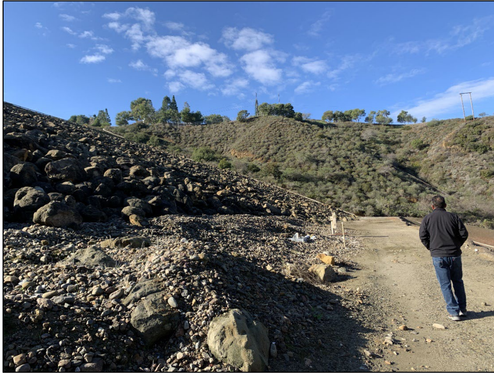
Photo 9) Downstream face looking towards the left abutment. Note upstream collector drain No. 1 and 2, and pneumatic piezometer vault box.
