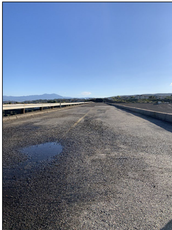
Photo 4) AC pavement cracking on crest.
