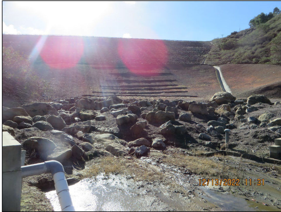
Photo 13) Looking at downstream slope at the toe of dam near the v-notch weirs and energy dissipator structure. Note minor normal seepage coming from dam toe.
