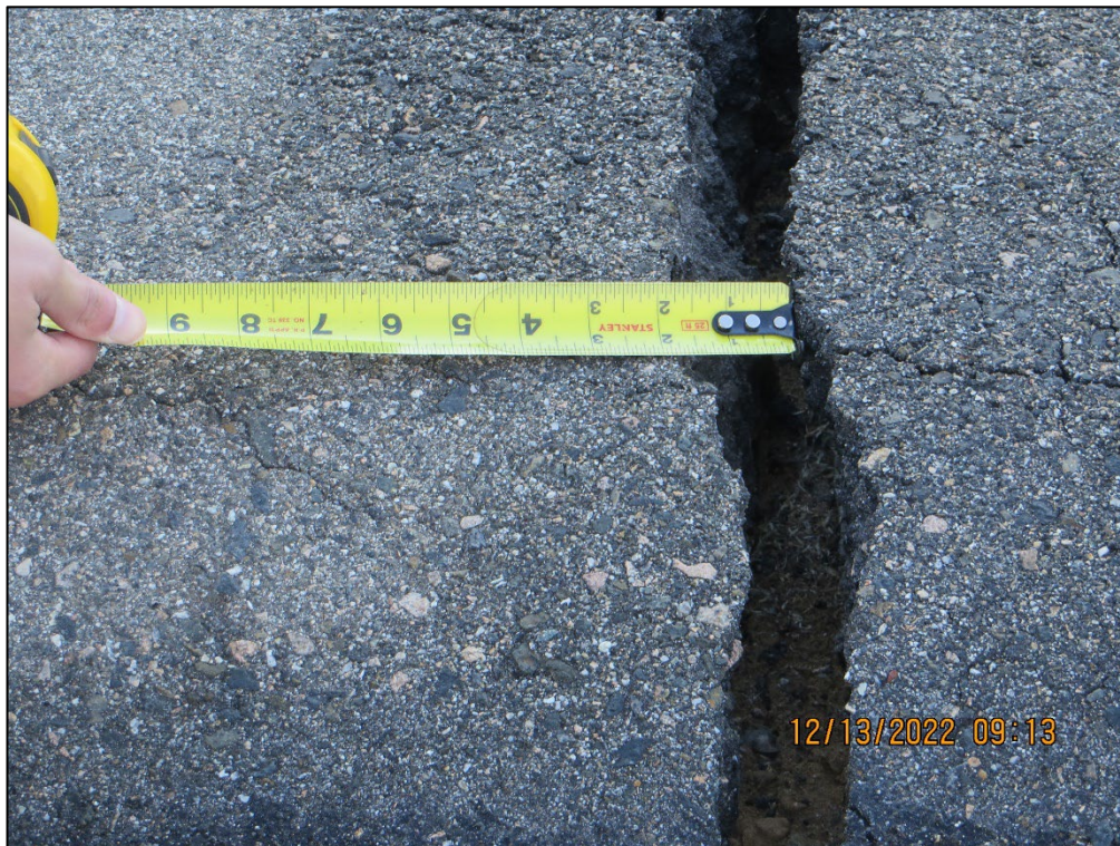
Photo 18) Approximately 2-inch-wide longitudinal cracking of reservoir liner at the left south end of the reservoir.
