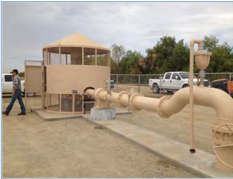
Figure 5. Kern Fan Project Recovery Wells will be Similar to Strand Ranch Wells
