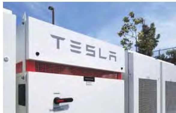
Tesla Battery Station
